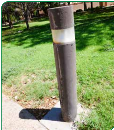
Light poles that are rusted and deteriorated and pose a danger of falling during a high wind event would be replaced using Bond C funds.
